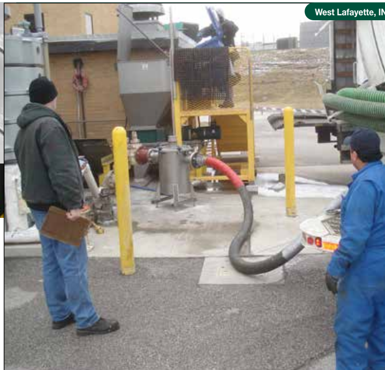
The Heavy Object Trap, helps this treatment facility turn grease into a renewable source of energy and get an immediate return on investment.
