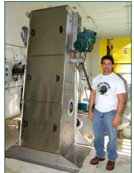
Anthony DeCicco, Superintendent of the facility, reports significant benefits with the new, multi-faceted Monster Separation System.
