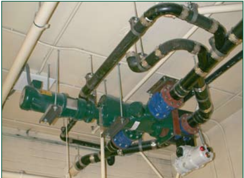
Here, a Muffin Monster hangs suspended from the ceiling, grinding solids coming from the laundry area of the jail.
