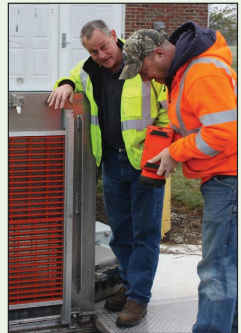
Village of South Elgin staff inspect the Muffin Monster and underground wet well.
