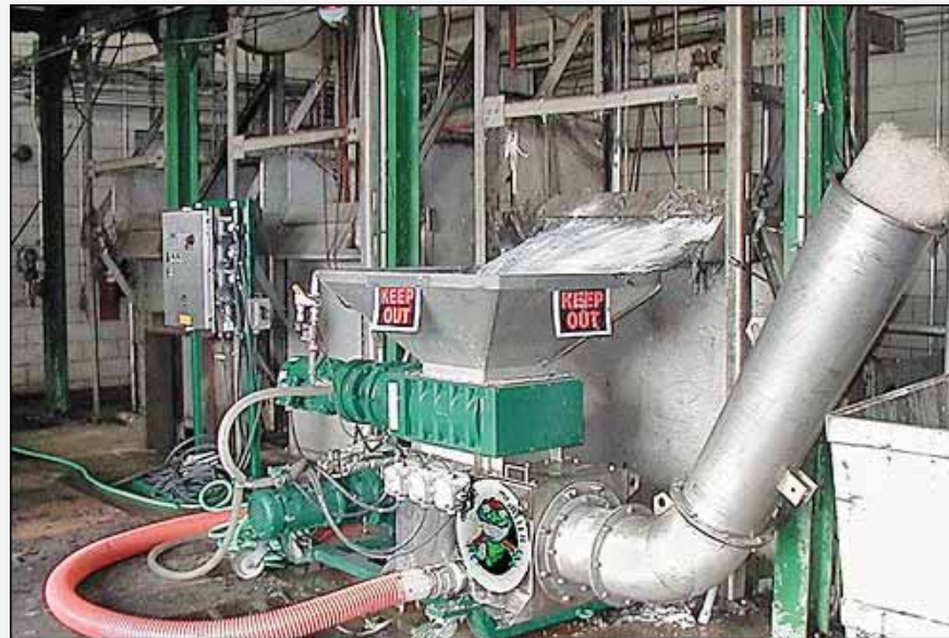
JWC Screenings Washer Monster Installation
