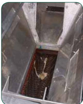
Muffin Monster grinder in a fish processing plant.
