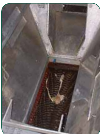
Muffin Monster grinder in a fish processing plant.
