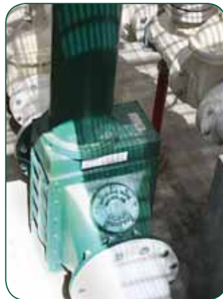
Macho Monster in-line sewage grinder in a jail.
